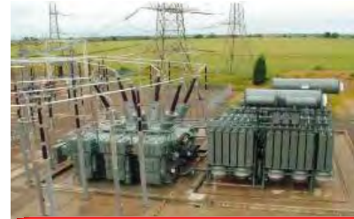
National Grid Phase Shifting Transfo.
